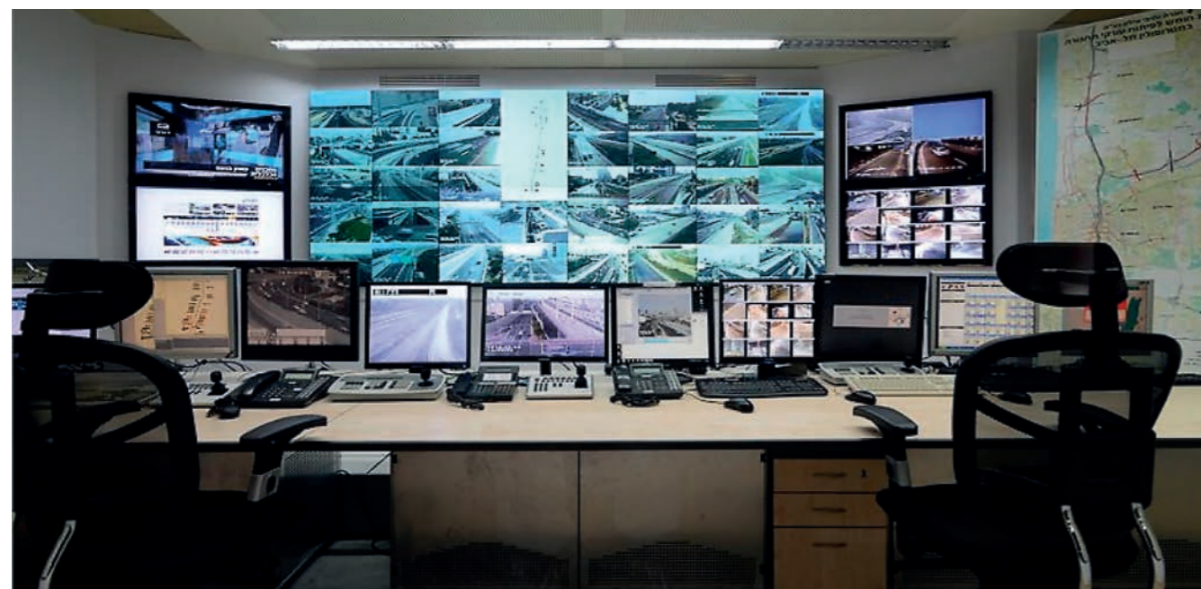
Figure 3.1.3. Example of Intelligent Traffic Center cockpit
